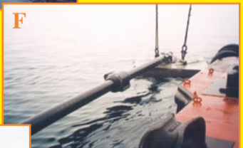
F: detail of the sinker (40 tonnes in air) linked to the metallic structure
