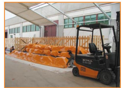
Dispatching the barrier
